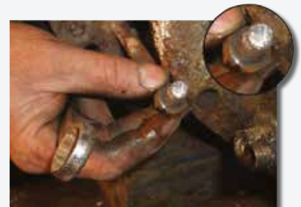
...which can lead to broken bolts.
